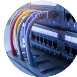
Data Center Compute
